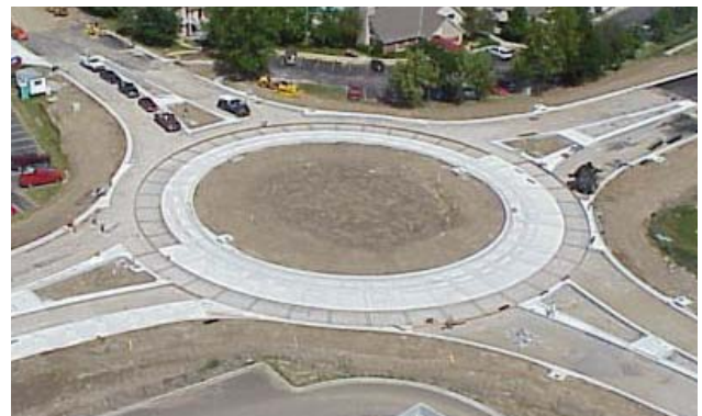
Figure 4. Inner ring complete, second ring under construction. Note the dowel baskets laid out in the circular portion, for the second and third rings.
