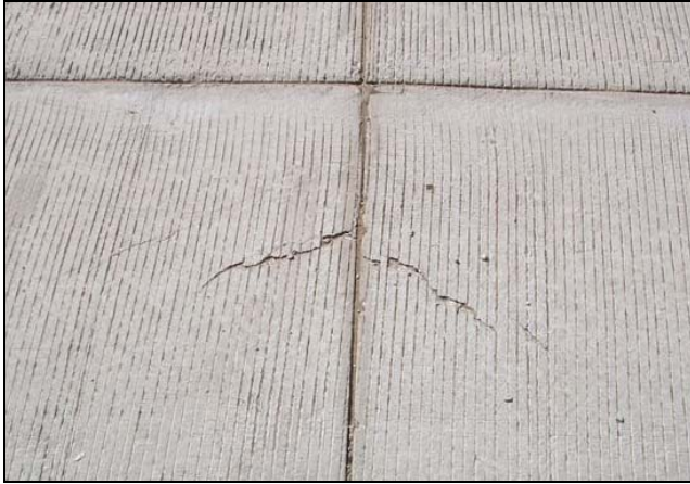
Figure 2. Photo of actual crack pattern from subject project. (NOTE: photo taken looking from driving lane toward shoulder).
