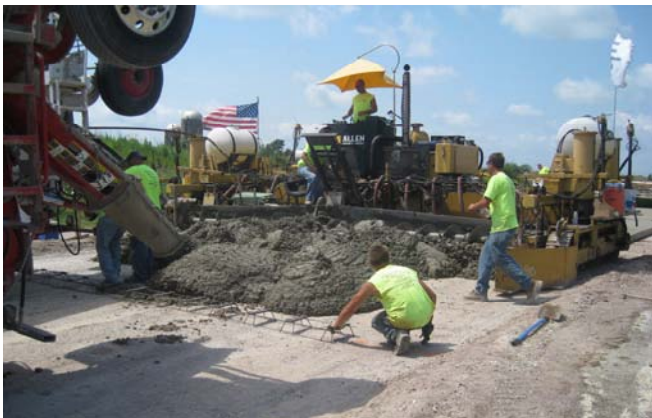
Figure 8. Slipform paving an industrial pavement that includes tapered plate dowel baskets. Note that the pavement was 8 in. thick and the dowel baskets were positioned just in front of slipform paving operations, allowing the prepared subgrade to be used as a haul road. [photo courtesy of PNA Construction Technologies, Inc.].
