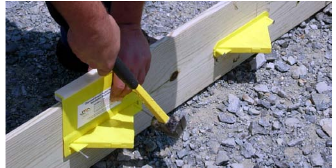
Figure 6a. Installation of a diamond plate dowel pocket former on wooden construction joint form [photo courtesy of PNA Construction Technologies, Inc.].
